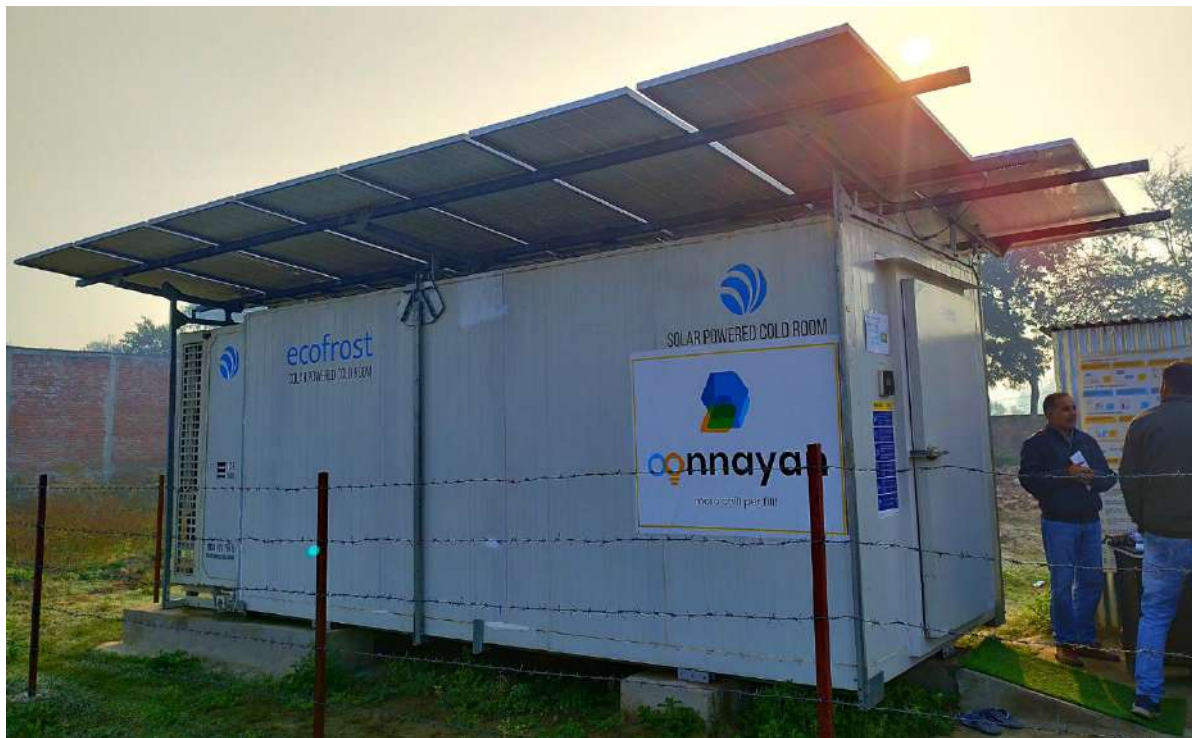
A solar cold storage in Bahraich district, Uttar Pradesh. These 5 MT cold rooms can store 30+ types of perishable produce, thereby achieving 400% higher shelf life.
